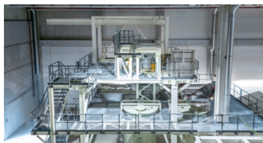
Figure 5 - Part of the Integrated LiB Plant installed by Primobius
